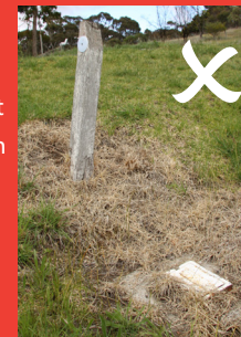
Faded post Overgrowth
