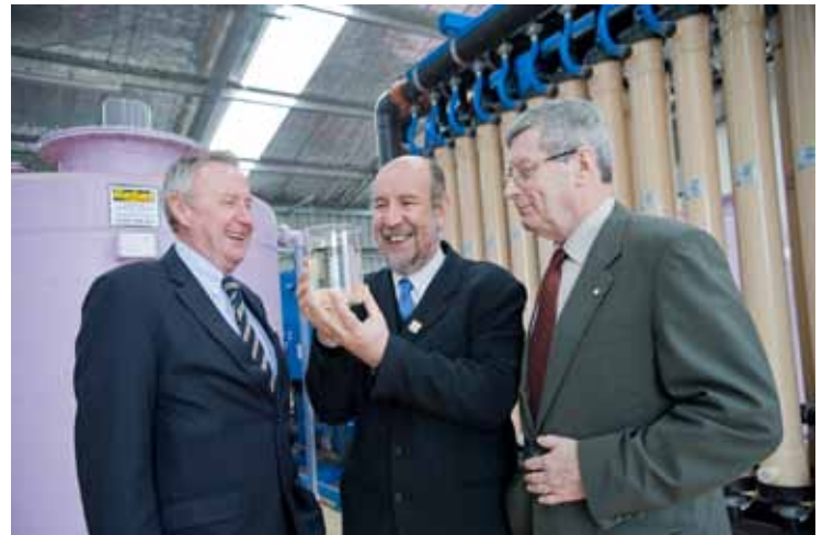
(L to R) John Wilkinson, Managing Director Western Water, Don Nardella, Member for Melton and Terry Larkins, Chairman Western Water examine Class A recycled water produced at the newly opened plant at Melton. Behind them is a bank of microfiltration tubes.
