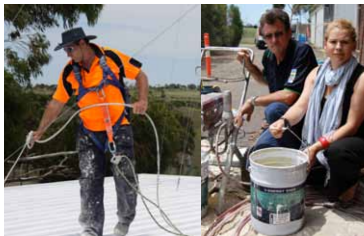
A contractor applies paint to the roof at Sunbury Recycled Water Plant as Team Leader Gerard Barry and Manager Renewable Resources Stephanie Gillespie observe.
