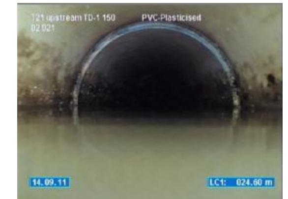
High level due to siltation
