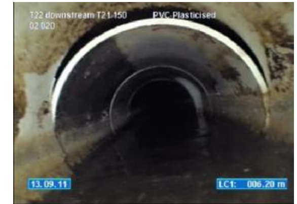
Radial Displacement, Partial Pipe Collapse
