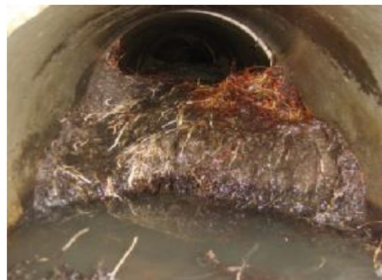
Blockage Due to Tree Roots
