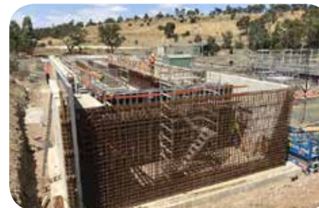
Photos above: Construction of the membrane tank. Photos taken in November (top), December (middle), January (bottom).
